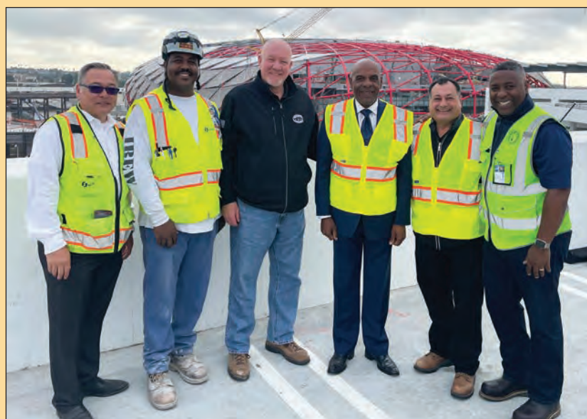
From left to right: Ron Watanabe, SASCO Superintendent, Darren Walton, MC3 Graduate and 2nd year IBEW 11 Inside Wireman Apprentice, NABTU President Sean McGarvey, California State Senator Steve Bradford who authored the bill to help create Intuit Dome, Ernesto Medrano, the new head of the LA/OC Building Trades Council, and Shomari Davis, IBEW 11 Business Representative in District 1 South.
