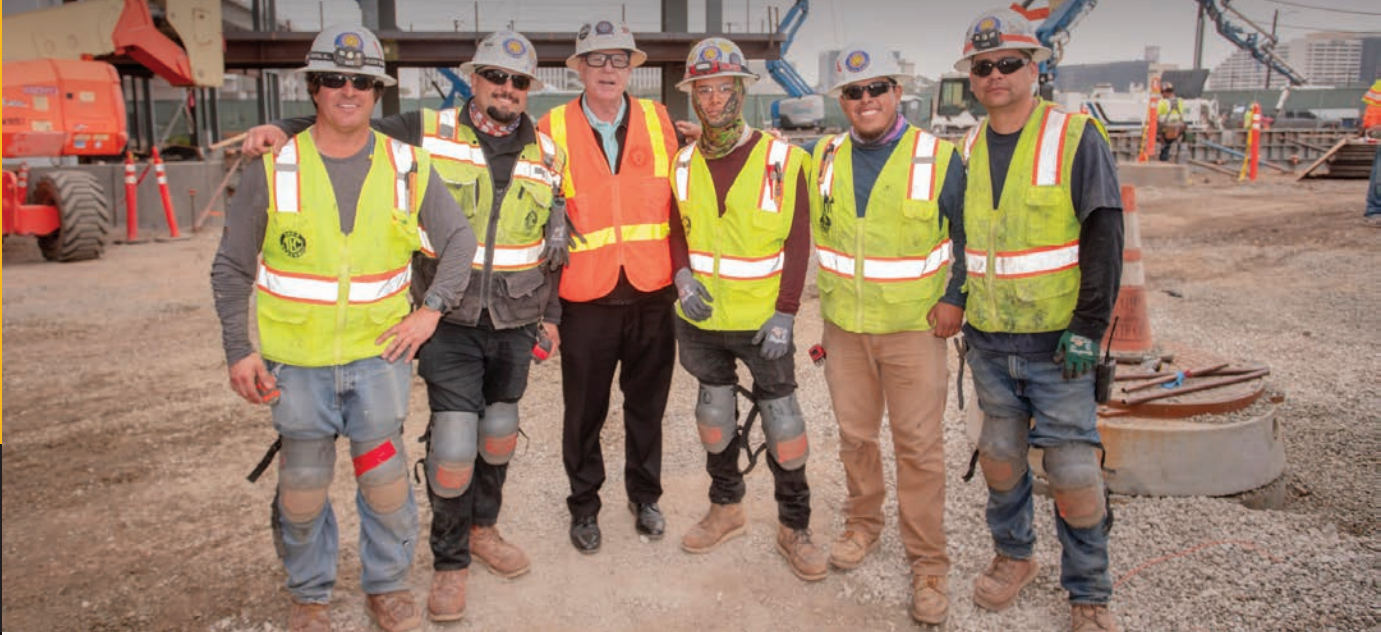
IBEW 11 Business Manager Joël Barton (orange vest) joined the Local 11 crew at LAX where union brothers and sisters are building a state-of-the-art transit hub that will transform how millions of passengers will get to and from the airport.
